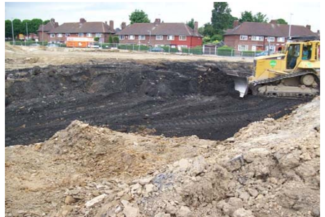
Coal close to the surface being extracted as part of ground works: prevents sterilisation and effective method of remediating unstable ground caused by former coal workings
