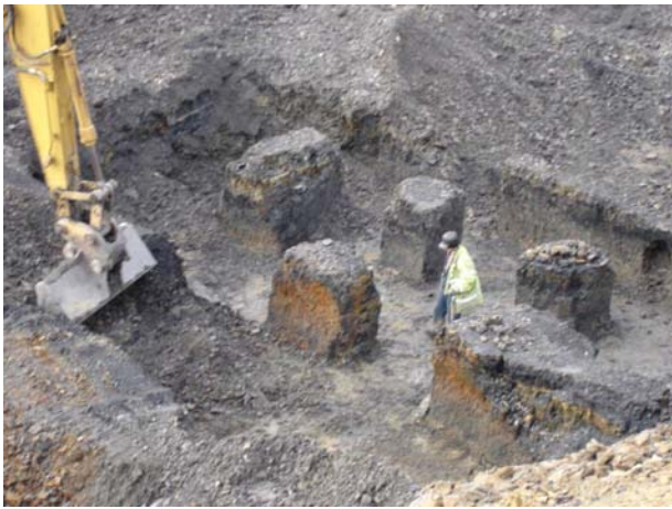
Pillars of coal being extracted as part of ground works: prevents sterilisation and effective method of remediating unstable ground caused by former coal workings
